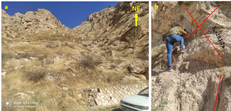
Fig. 10: Station (5): (a) Front view of the station showing part of the retaining wall destroyed by blocks falling from the top of the station, (b) Discontinuities in the station.
